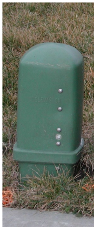
Cable TV Pedestal
