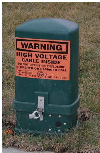
Low Voltage Dome
